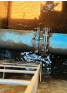
A severe pipe leakage at the Y-piece.
